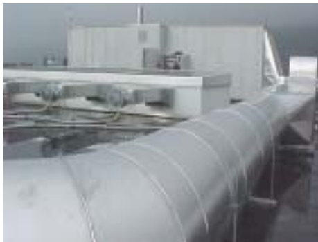
Overall view of system
