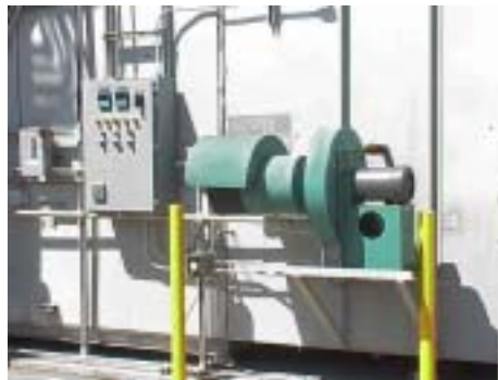
Combustion Air Blower/Filter and Control Panel for one of three units.
