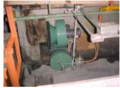
Eclipse ImmersoJet Burner on E-Coat Line
