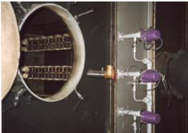
2 of 3 burner rows visible through access port.
