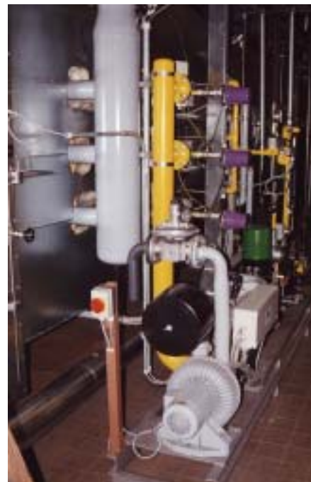
Primary air supply and gas manifold with pilot/cooling air blower and valve trains.
